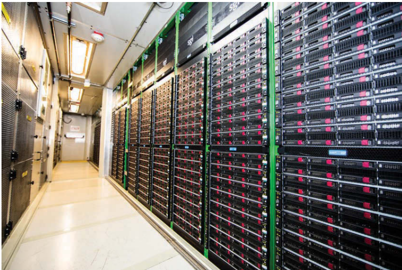
Figure 4. Racks of computers or “rack” servers in a data center.
